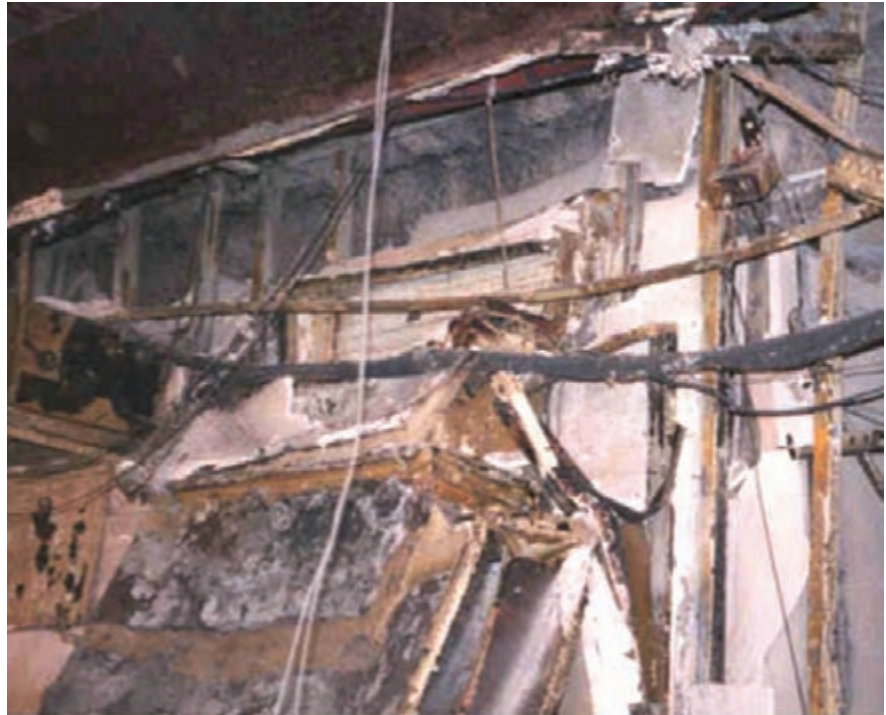
Figure 5: Fire Damper Performance in WTC 5
